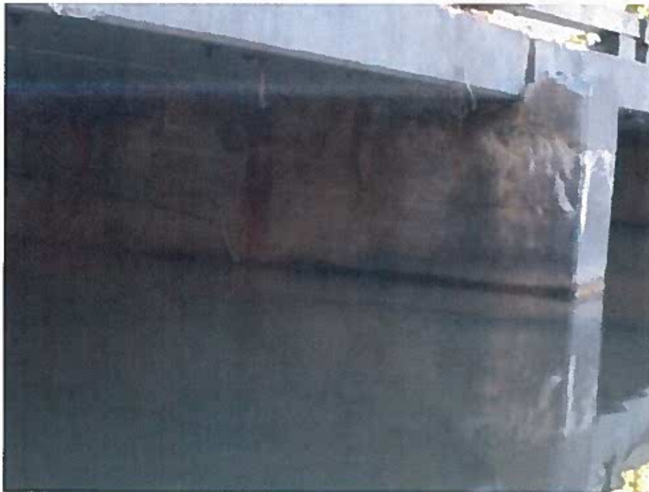
Pier 4 – Spalling with Exposed Reinforcement
