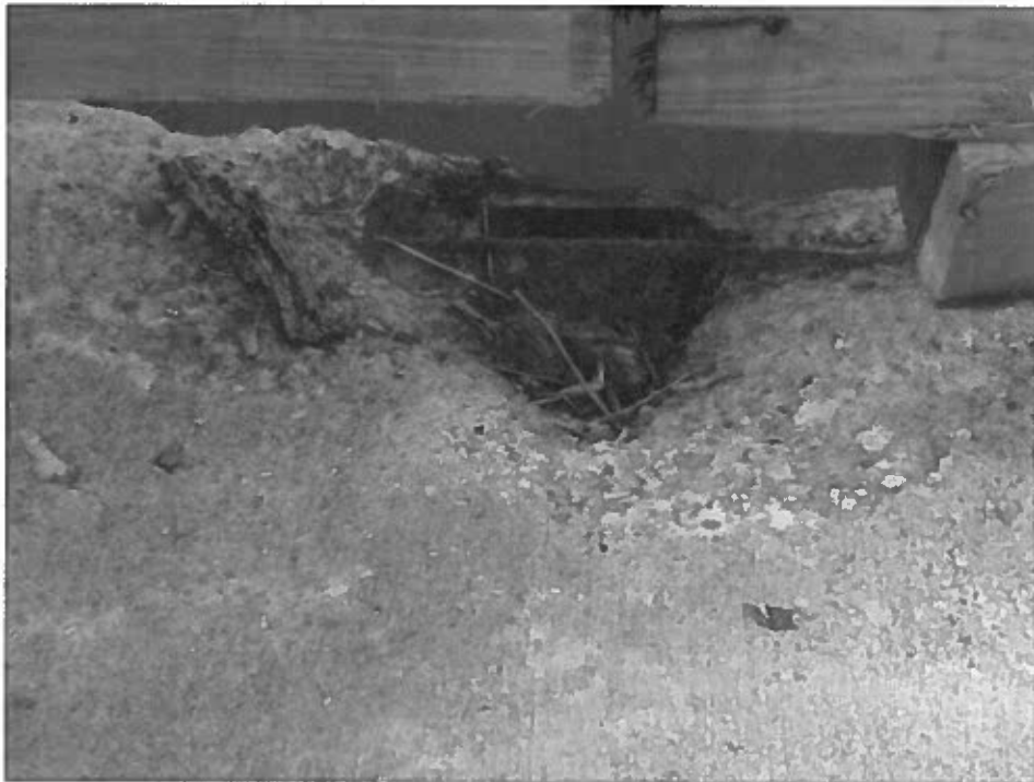
Beam 5, Span 3 – Spall with Exposed Reinforcement at Lateral Tension Rod Location
