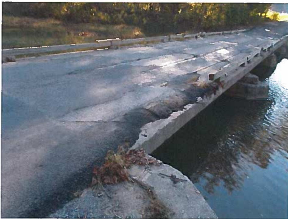
Missing Curb, Right Side of Span 1
